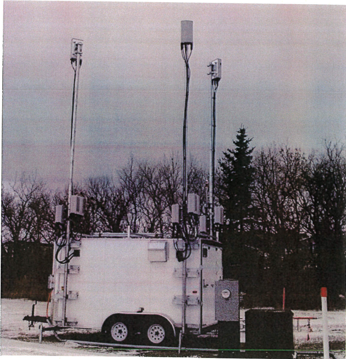
Temporary "Small Cell on Wheels" (SCOW) Trailer
