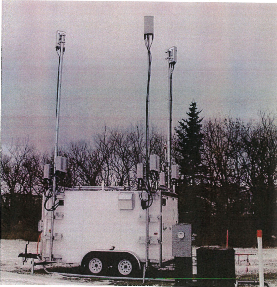
Temporary "Small Cell on Wheels" (SCOW) Trailer
